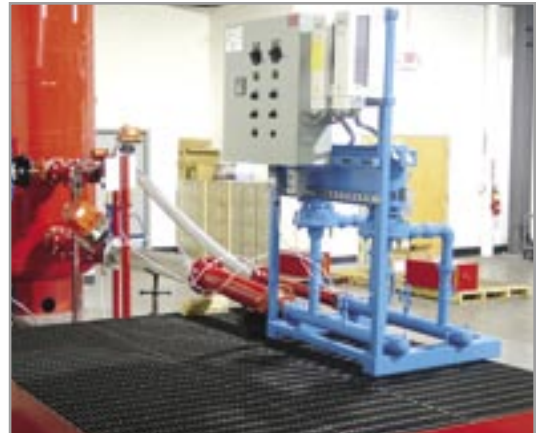
Booster System Undergoing Testing.
